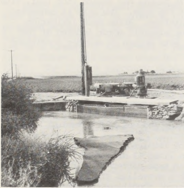
FIGURE 1-6. This booster pump takes water from the canal and pumps it into aluminum mainline pipe which delivers it to sprinkler heads in the field.
